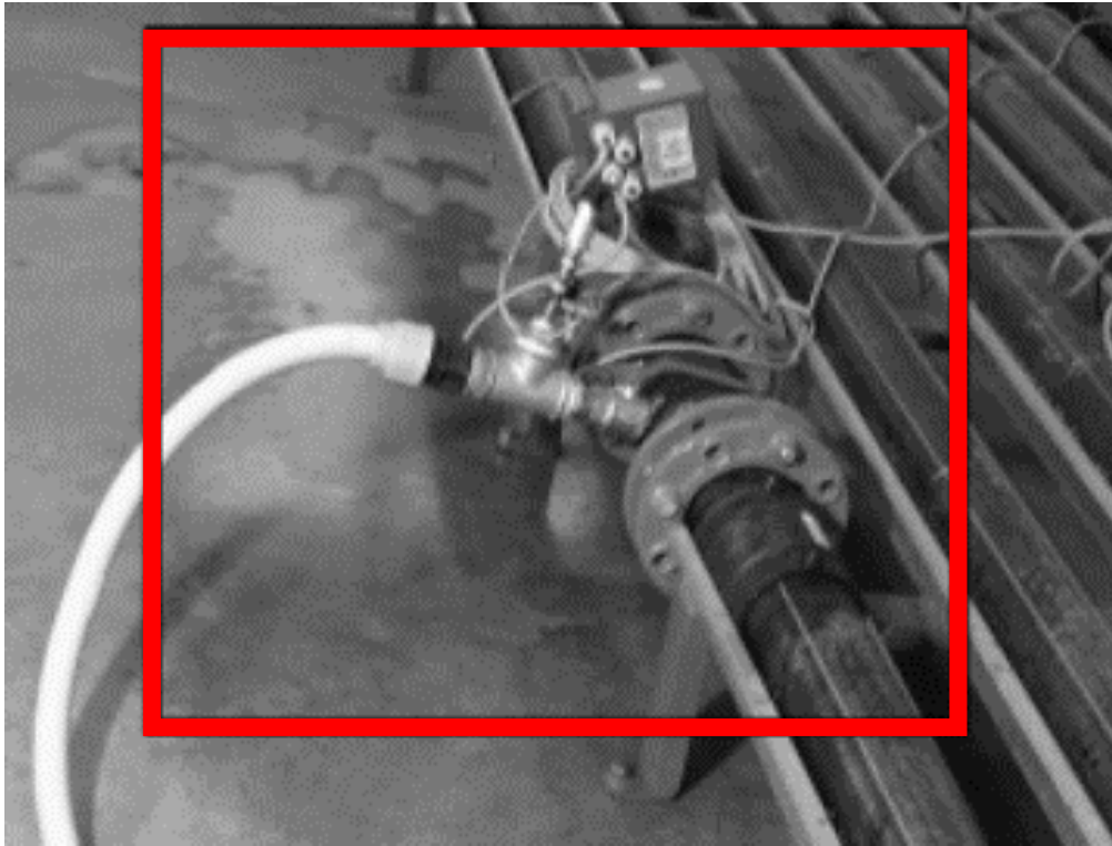
Valve directly attached to pipe - Meniconi et al. (2011)
