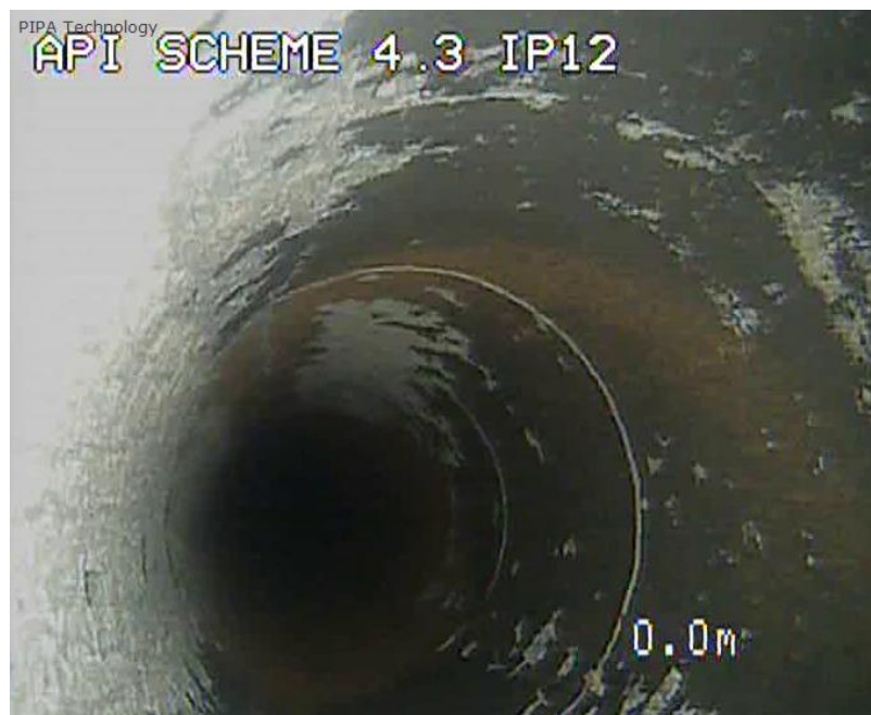
Cement lined pipe
