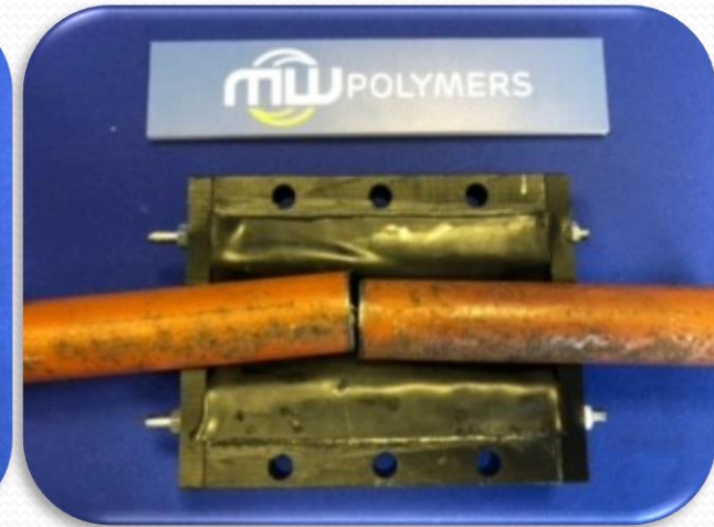
Fitted clamp on a cracked pipe
