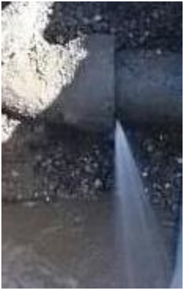
Failed joint seal
